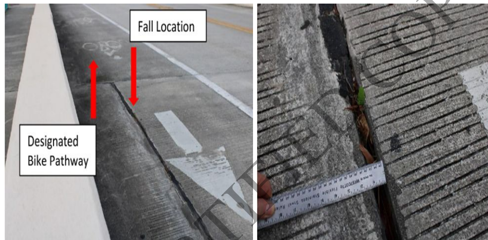
Photographs of the fall location and the "gap" in its state of disrepair
